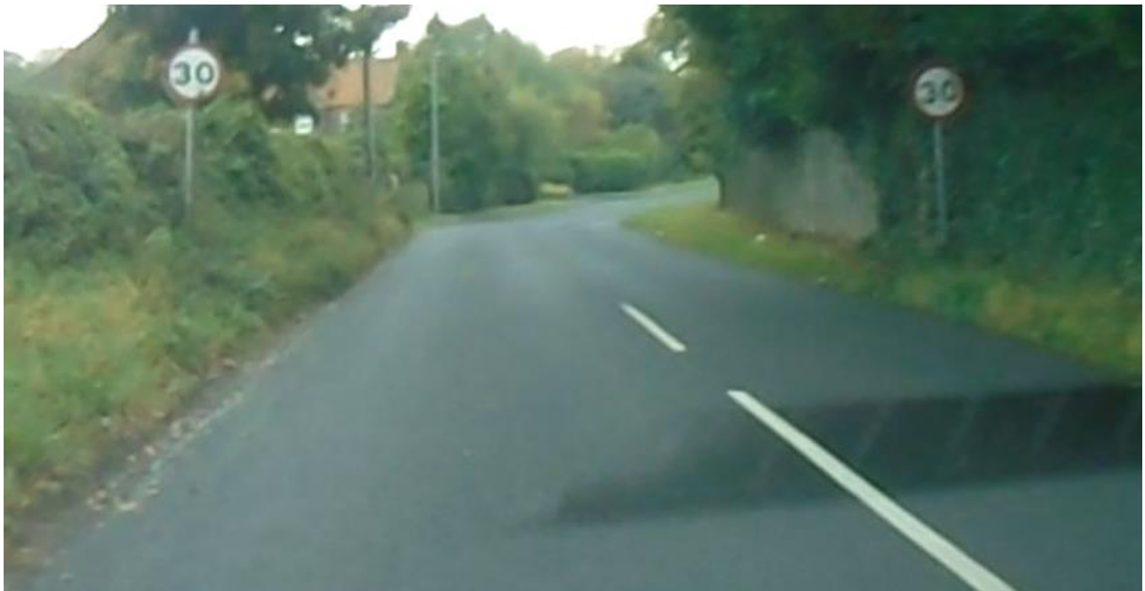
Photo 17 - Example of removal of carriageway centre line at B1339 southbound entrance to Lesbury Village
